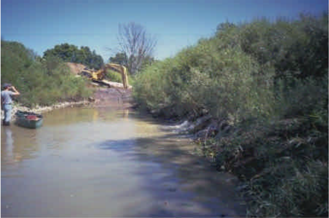
Photo 7. Reach BEAR 4. Pipeline construction has blocked the channel and the flow is being pumped around the site and down the bank (center).
